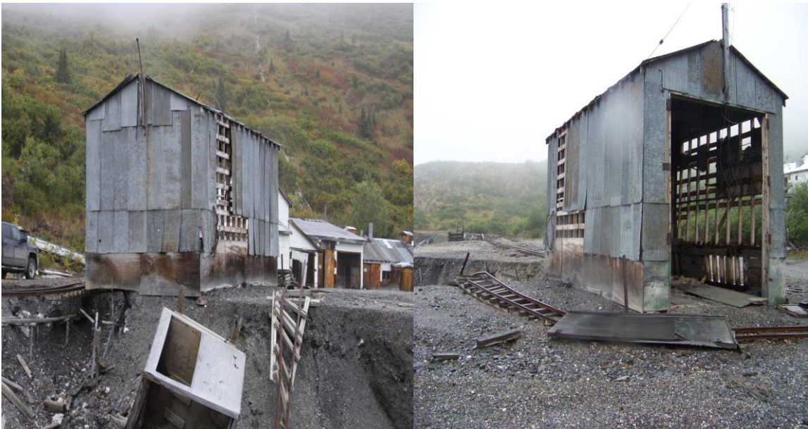
Picture 1. One of the buildings on the verge of collapse on the Keno 700 site and old rusted ore cart rails surrounded by piles of gray objects lying around all kind of scattered crude equipment used to work the mines.
